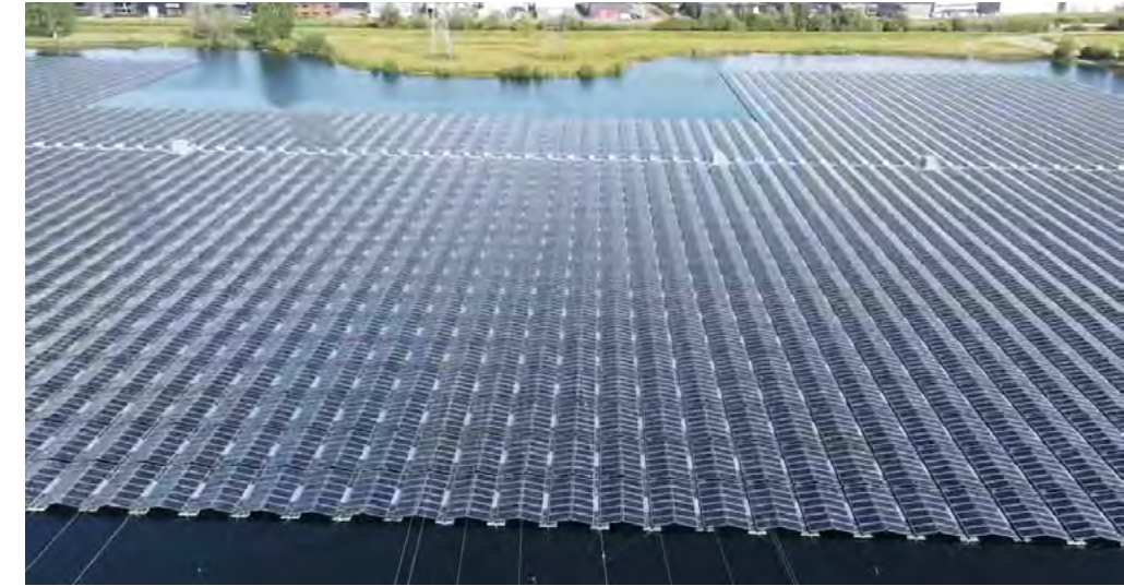
Sekdoorn solar park (15 MW, Netherlands)
