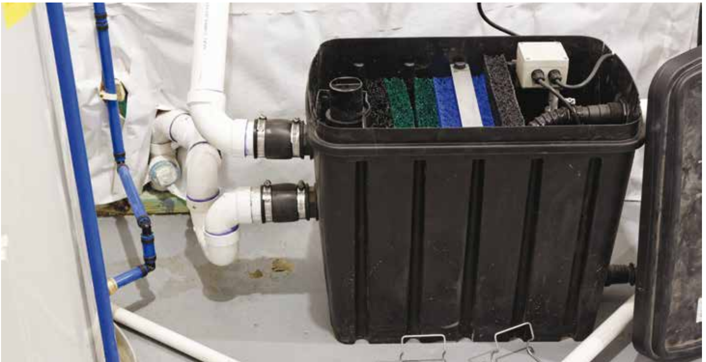
Second Life. Graywater from bathroom sinks, showers and the washing machine passes through the multiple filters of the Aqua2use system before being stored in Rainwater HOG tanks located under the deck.
