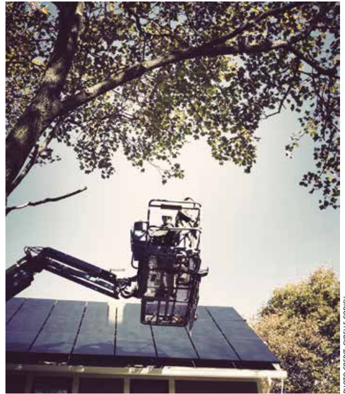
Power House. An 8.1 kW photovoltaic array from SunPower and Enphase microinverters helps this 114-year-old Michigan home produce more energy than it consumes.
