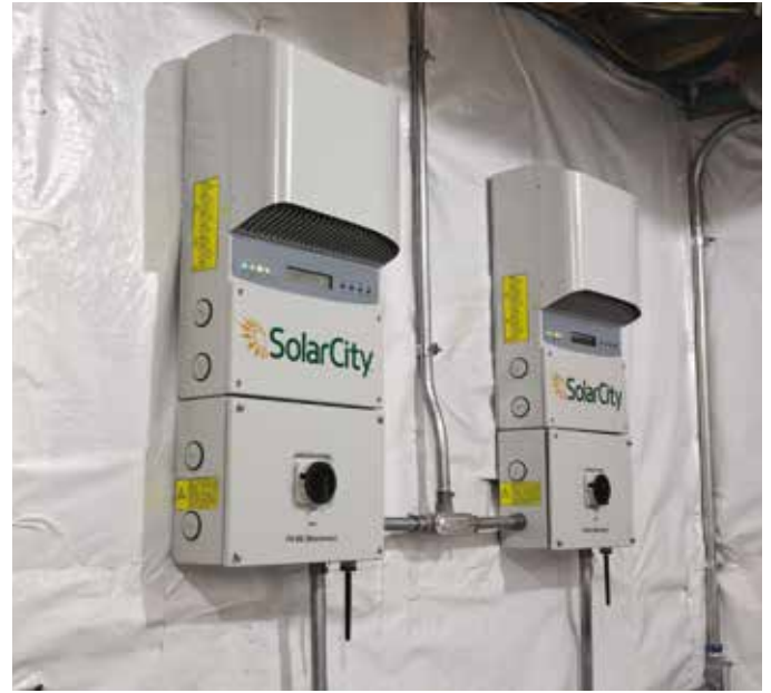
Going Below Zero. A 9.95 kW array from SolarCity helped the PureBlue Home earn its -1 HERS rating.
